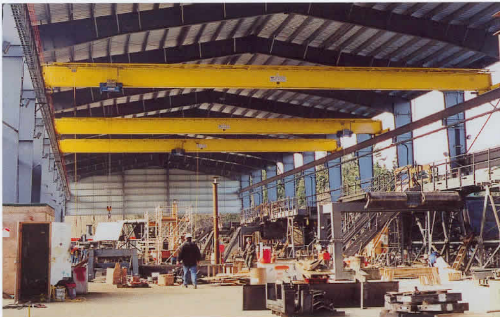
These single girder cranes were installed at the casting yard that produced massive concrete girders for the multi-billion dollar Skytrain extension in B.C.'s Lower Mainland. All the cranes have 84-foot wide spans.
