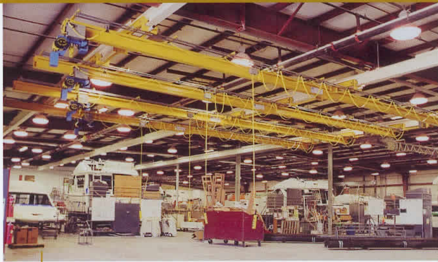
These four under-running multi-span cranes were designed for a boat-builder in the U.S. The girder is hinged at the point of maximum roof deflection to ensure the crane does not lose contact with the rail on either side.
