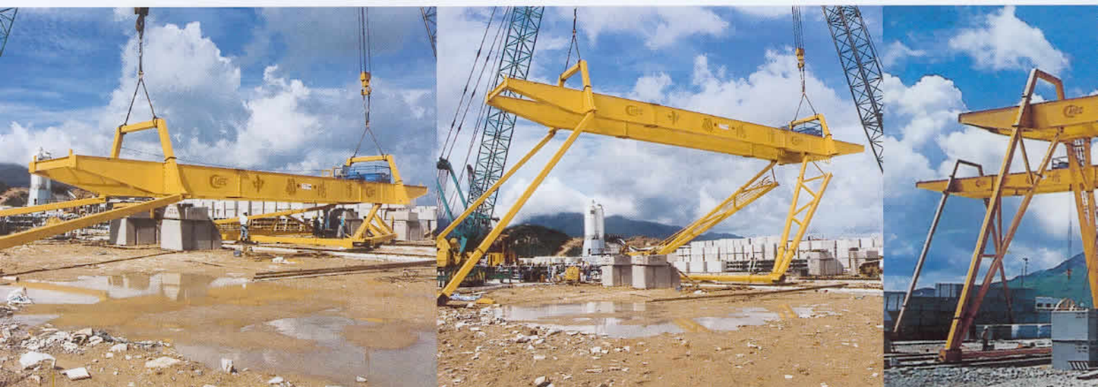
This series of shots demonstrate the versatility and ease of erecting a gantry crane. The crane had been assembled on the ground and lifted into place. Once erect, all that was required to complete
